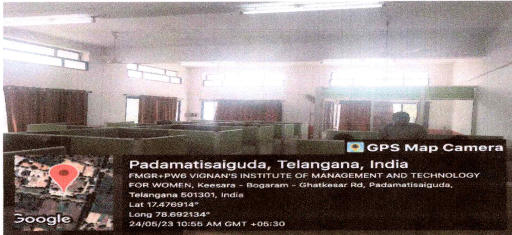
Use of LEDs in Staff Room
