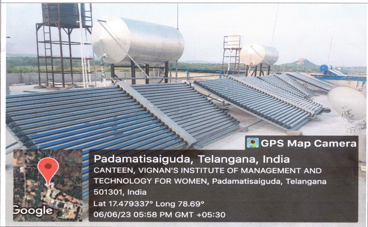
Solar Power Panel
