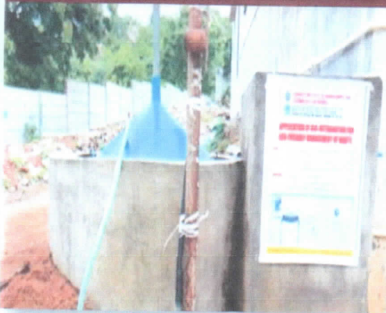
Bio Gas Plant
