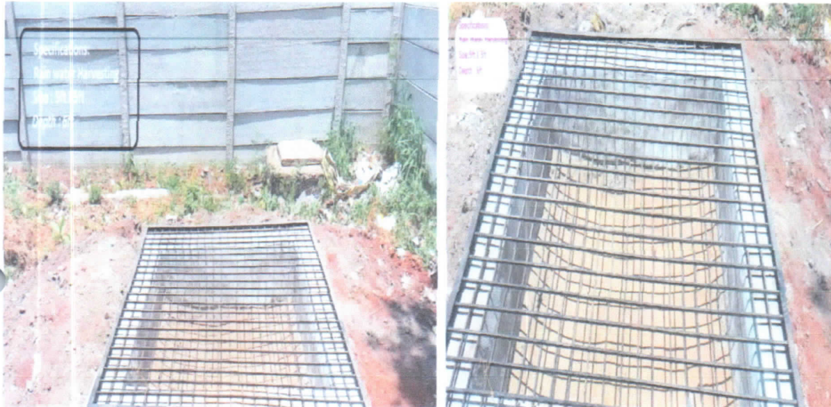
Rain Water Harvesting Facility
