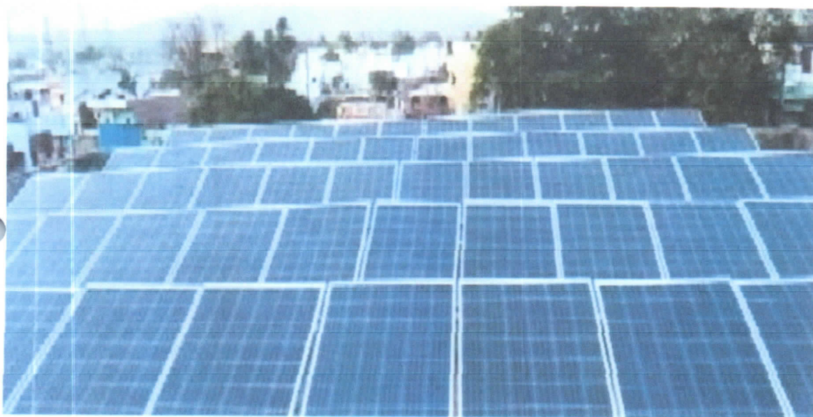
Solar Power Panel on the rooftop with a capacity of 50kW
