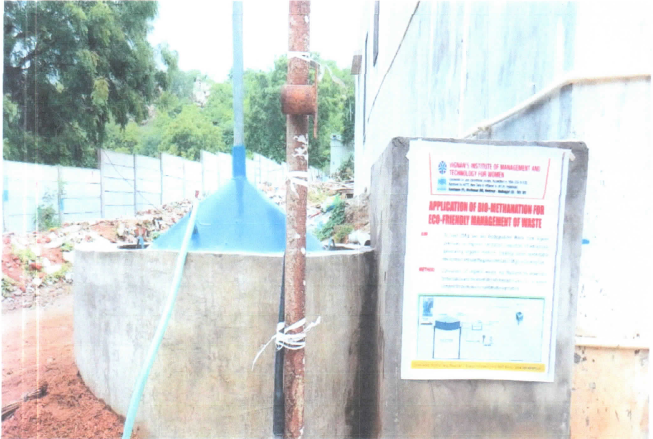
Bio- Gas plant
