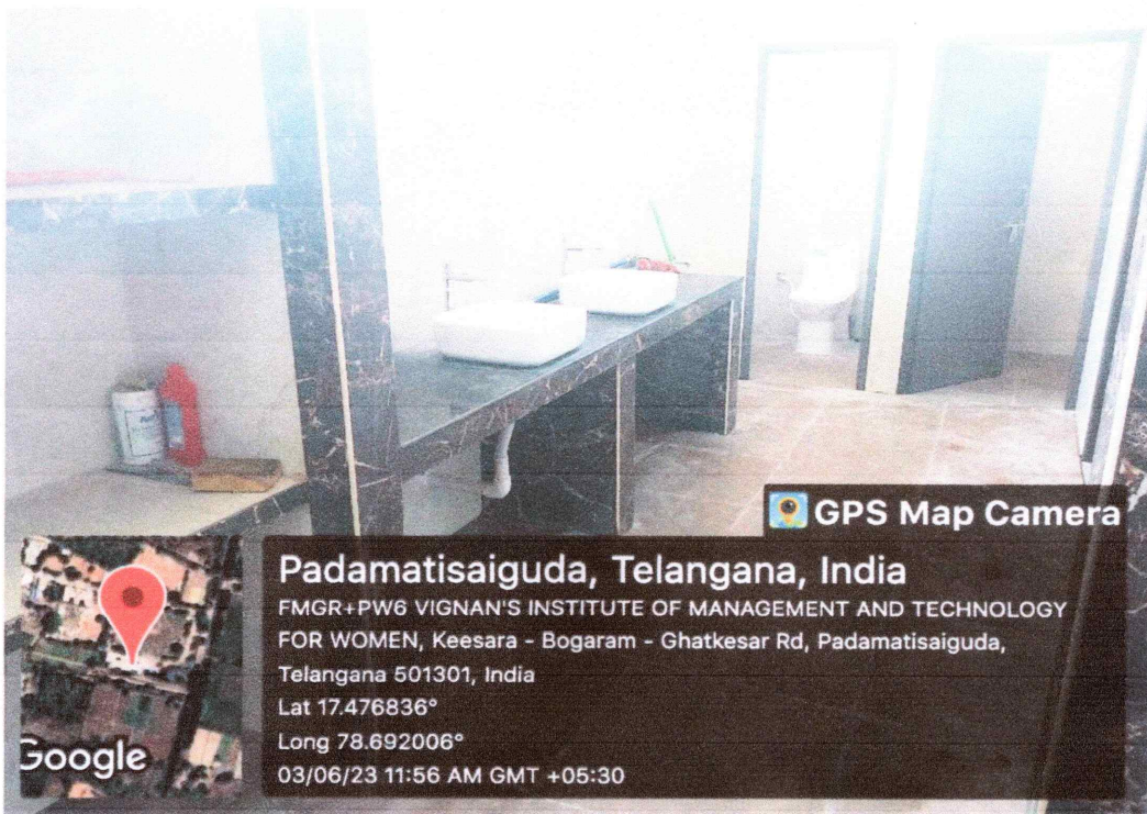
Disable friendly wash room
